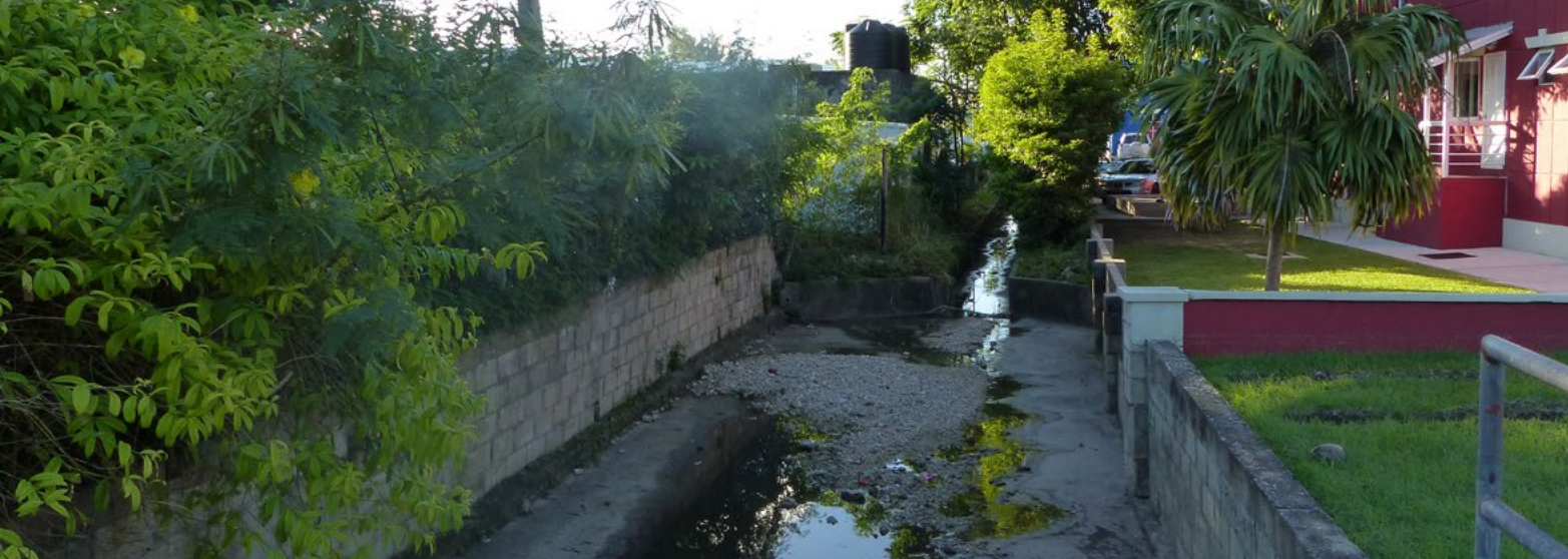
> Channelised gully outfall prone to flooding
