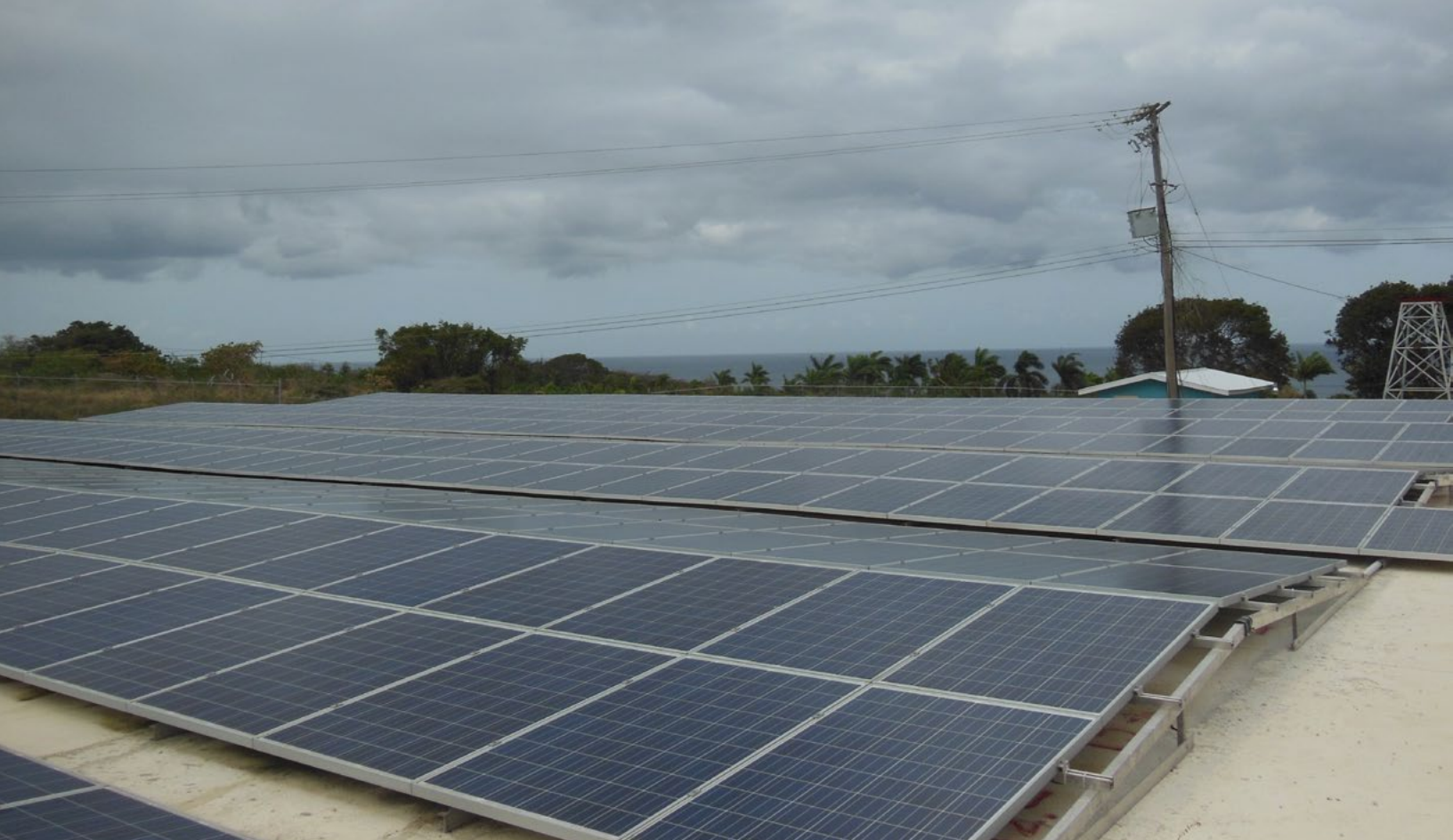
➤ Solar powered BWA pumping facility, St. Peter
